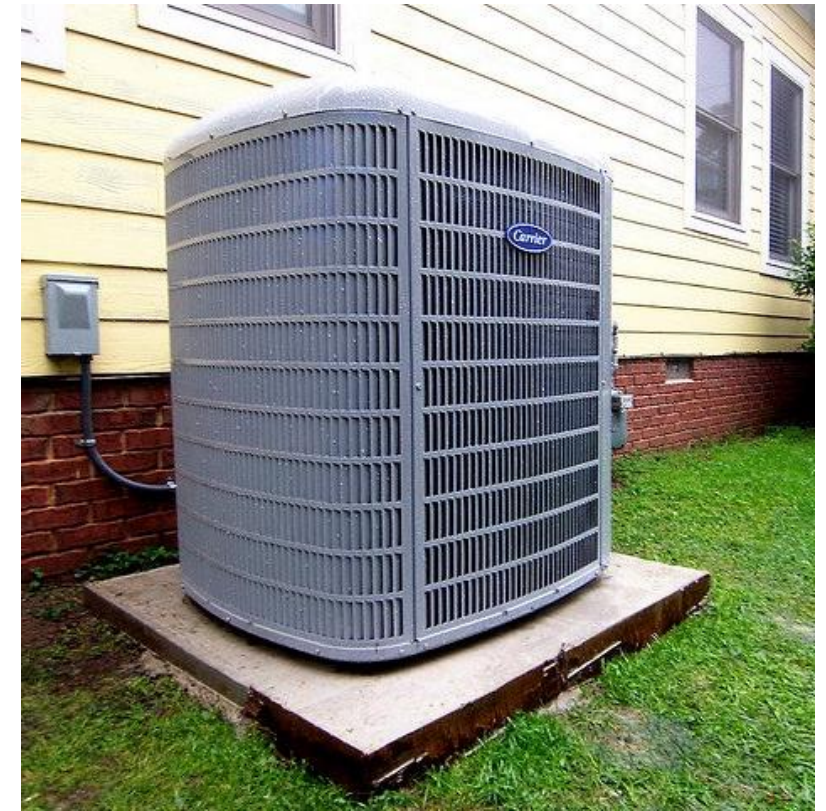
Remote Outside Condenser
