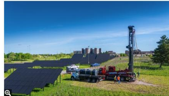
The university conducted its first geothermal well test drill near the Baker Chilled Water Plant in May 2025. Photo: Douglas Levere
